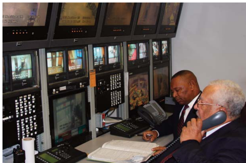
Special Security Officers Reginald Fortune (with phone) and Stanley M. Booker operate the control room.
